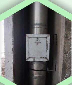
GARBAGE CHUTE SYSTEM
